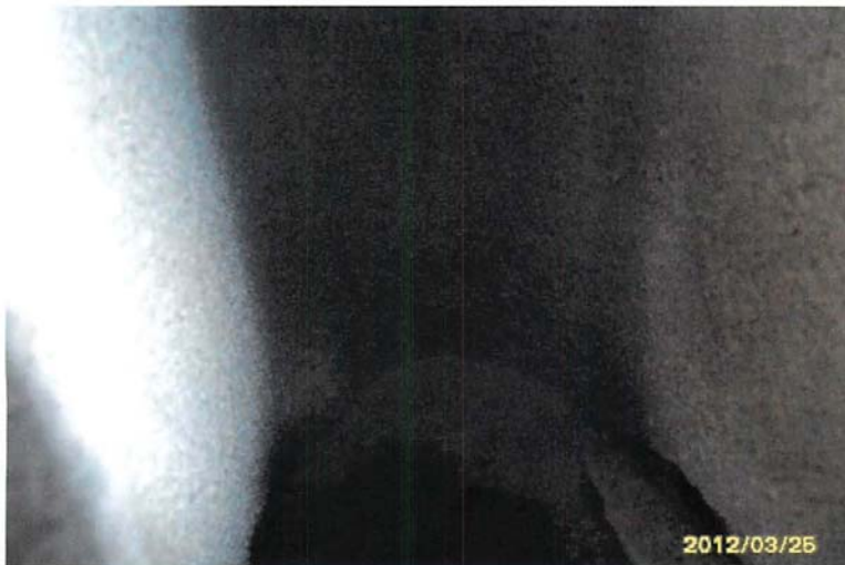
Interior of concrete block at exterior wall of former Highway Garage. There was no Vermiculite observed inside block walls.
