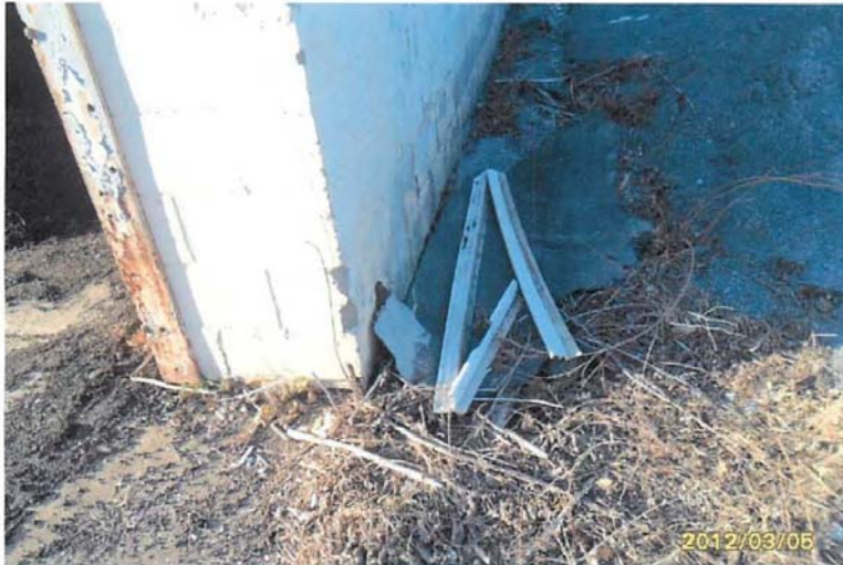
Asbestos roofing debris at exterior of former Highway Garage.
