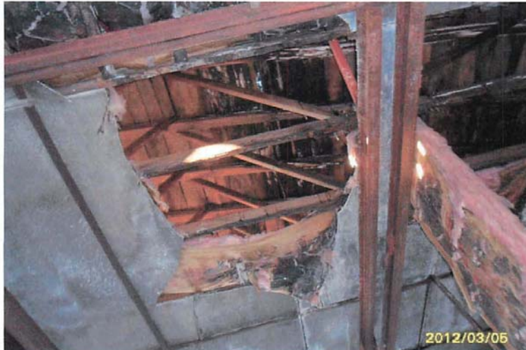
Damaged ceiling at interior of former Highway Garage.
