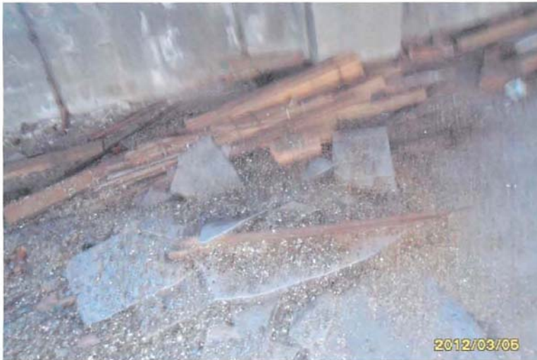
Asbestos Transite ceiling panels and presumed asbestos Vermiculite ceiling insulation debris at interior of former Highway Garage.
